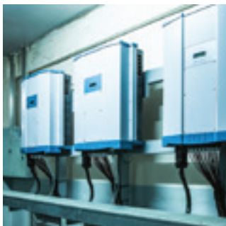
PV Energy Storage Systems
