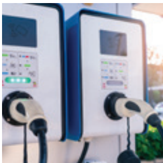
EV Charging Stations
