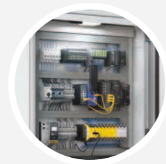
Control panel technology, DIN rail terminal blocks
